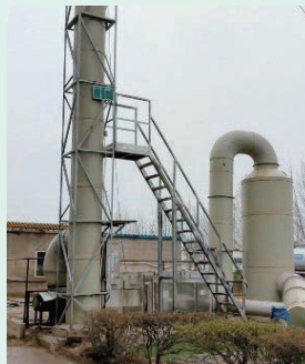
Waste Gas Treatment Equipment of the Sewage Tank—Dispose of Foul Smell of Sewage 污水池的廢氣處理設備 — 處理污水臭味
