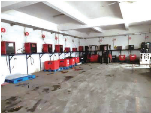
Forklift Charging Room 叉車充電間
